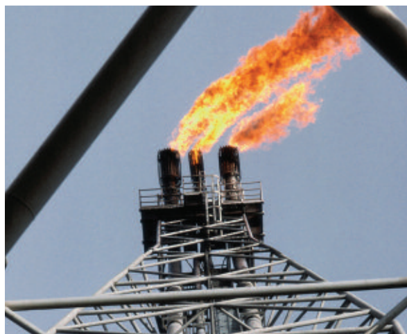
Today's refineries and chemical plants frequently burn-off waste gases in a flare line. Because both flow rates and gas compositions vary, the TA2 can be used to obtain relative flow indication.
